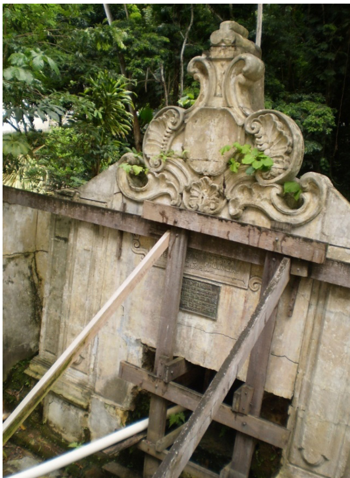
Figure 5. Degrading situation of the pediment built in the 18th century to identify the Tambiá Fountain, richly carved in limestone with baroque elements. Photo: the authors
