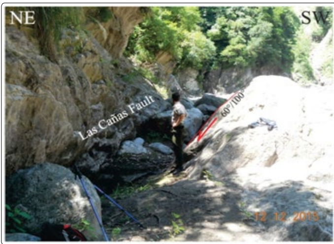
Figure 6. Las Cañas fault on the right riverbank of the Las Cañas River.
